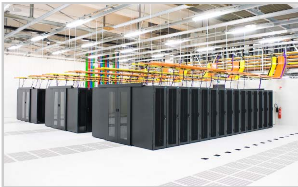
How green is your datacentre? Pictured here is Telecity's Condorcet datacentre - designed to be as energy-efficient as possible (Photo credit: Telecity)
